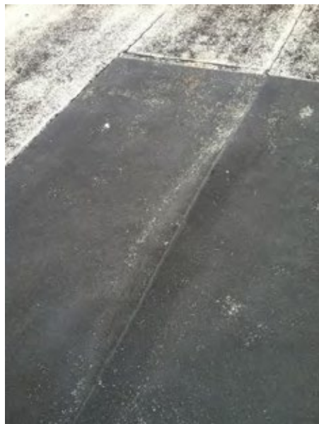
Photo 3 Bubble in Roof
