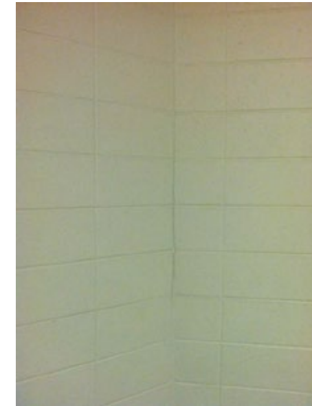
Photo 4 1974 Addition Stair Wall Crack
