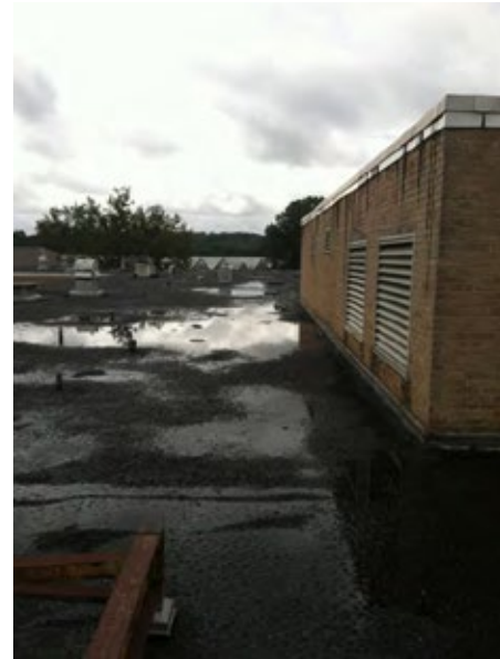
Photo 6 Water Ponding on Roof
